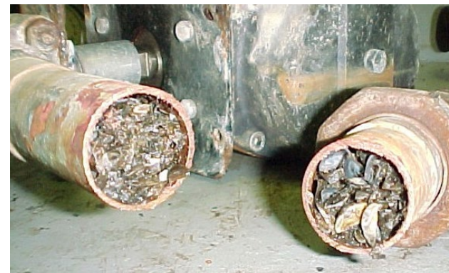
Source Water Impacts: Water pipe clogged with zebra mussels
